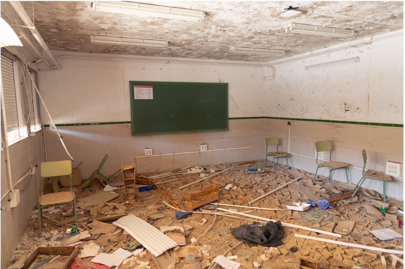
The Carme Miquel del Arrabal primary school in Algemesí (Ribera Alta county) still lies in rubble, pending demolition and reconstruction at the same location.
